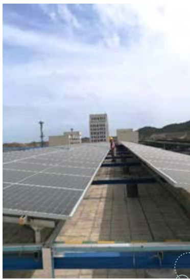
The photovoltaic power generation project (Phase I) of Xia Men Bay China Merchants Terminals Co., Ltd. was completed and put into operation during the Reporting Period.
